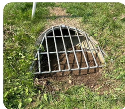
A culvert with a rodent guard gate and visible sediment accumulation
