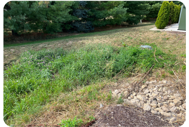
A poorly maintained facility bottom. Weeds have taken over and covered the outlet structure.
