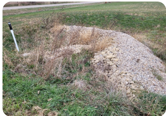
A stone weeper with unwanted vegetation growth
